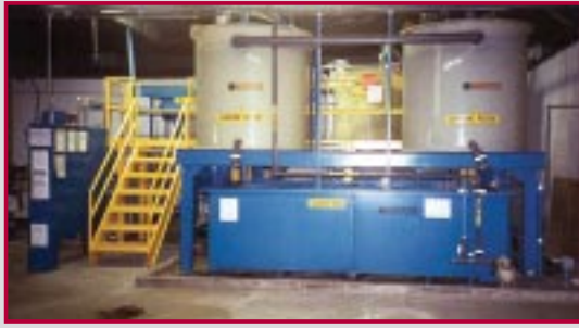
NAPCO WASTE WATER TREATMENT SYSTEM
